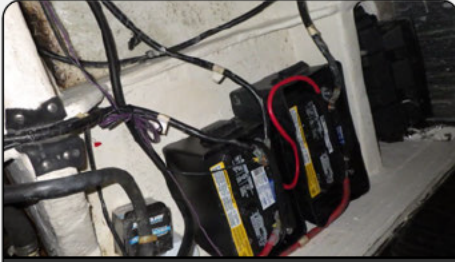
Photo 4: Port battery bank. No covers on terminals and on stbd battery a small black wire is sighted under large cable. No overcurrent protection within 7 inches.
