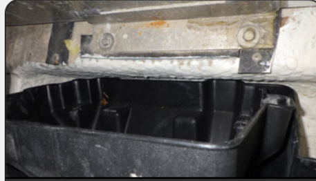
Photo 5: Battery cover not in place
