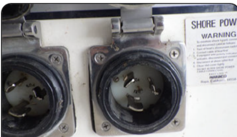
Photo 36: AC power inlets showing no evidence of arcing
