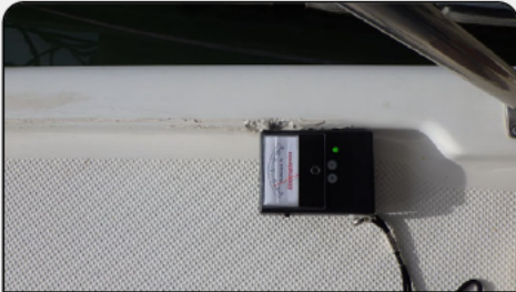
Photo 17: Poor quality repair but no water intrusion at this stage. Note slight crazing on toe rail on LHS of photograph
